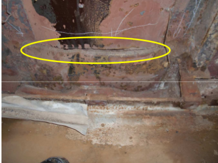
Horizontal cracks on front face
