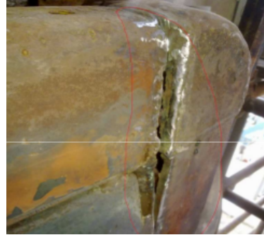
Cracks in the expansion joint flanges
